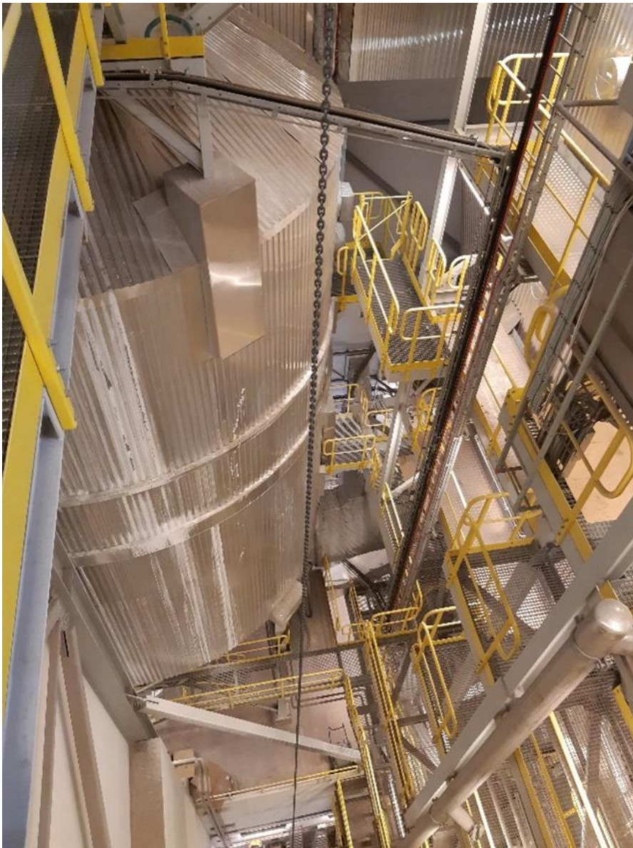
Figure 3. Flue gas treatment at Åmotfors waste-to-energy plant.
