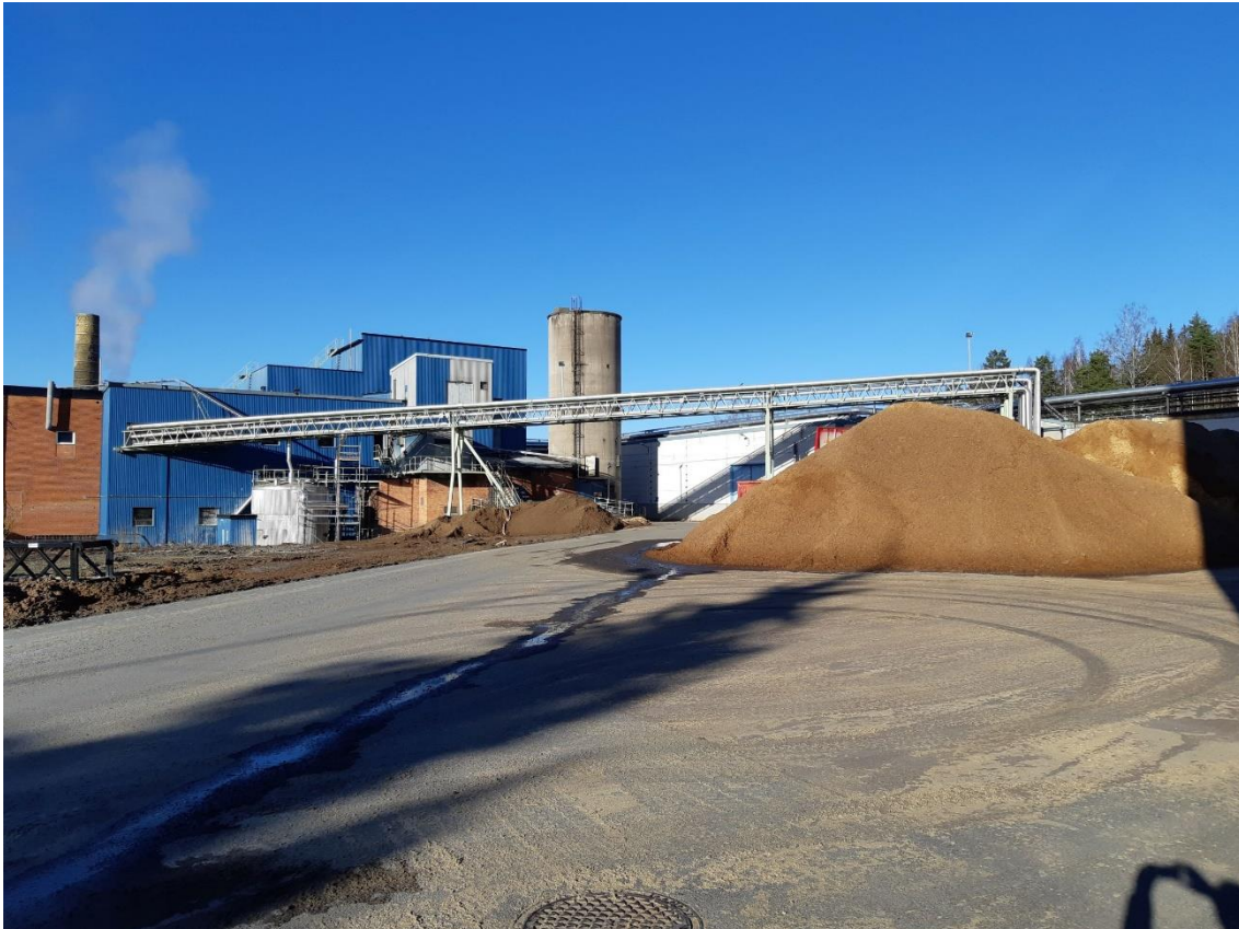
Figure 5. Pipe bridge for steam delivery to the paper mill.
