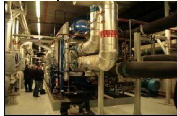
District cooling plant at Spittelau Incineration plant in Vienna.
