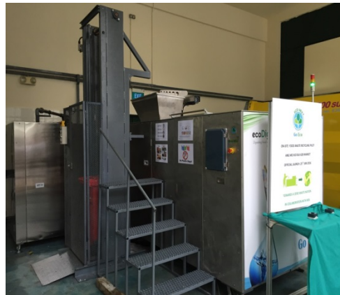
On-site food waste recycling machine at food centre
