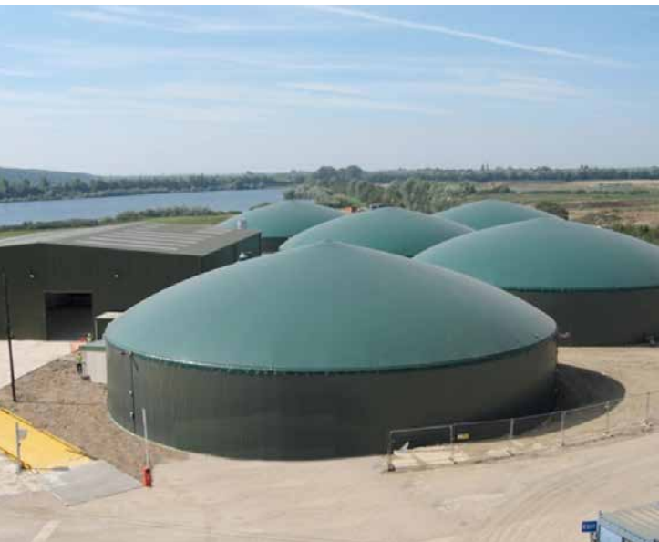
Figure 5: The Cassington AD facility in Oxfordshire, United Kingdom. The biogas plant processes source separated municipal and commercial food waste (Source: www.biogas.org.uk )
