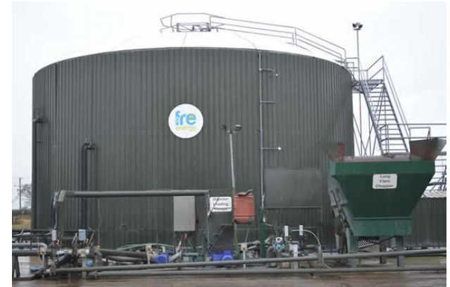
Lodge Farm Digester, Wrexham
