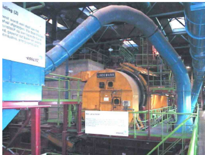
Figure 12. Waste pre-treatment at VAM plant.
