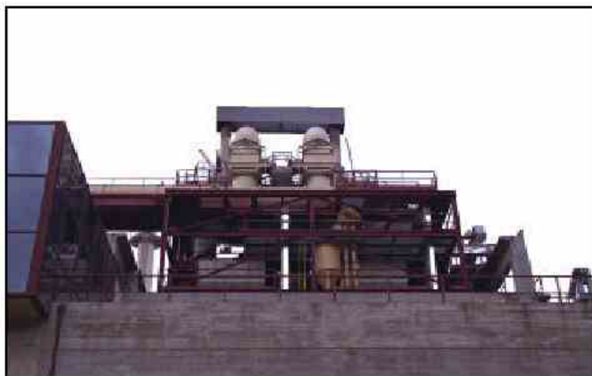
The 2 gasifiers at Gréve-in-Chianti
