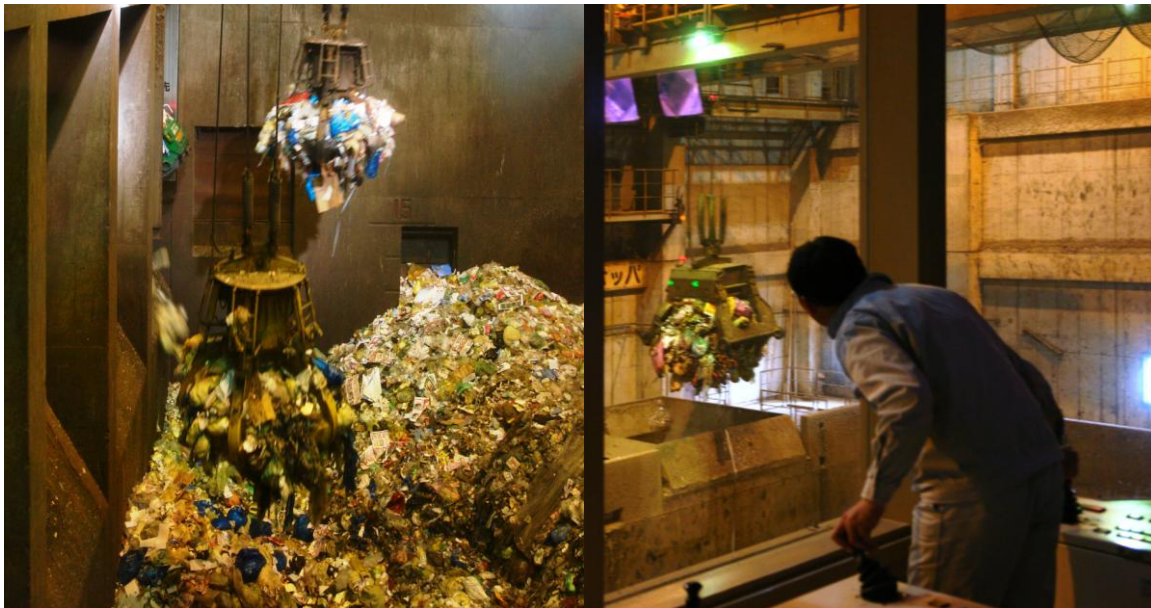
Figure 4.3: Waste bunker with two cranes mixing the waste (left) and filling the feeding hopper with a crane load of waste (right)
