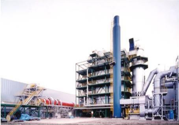
Takuma pyrolysis plant
