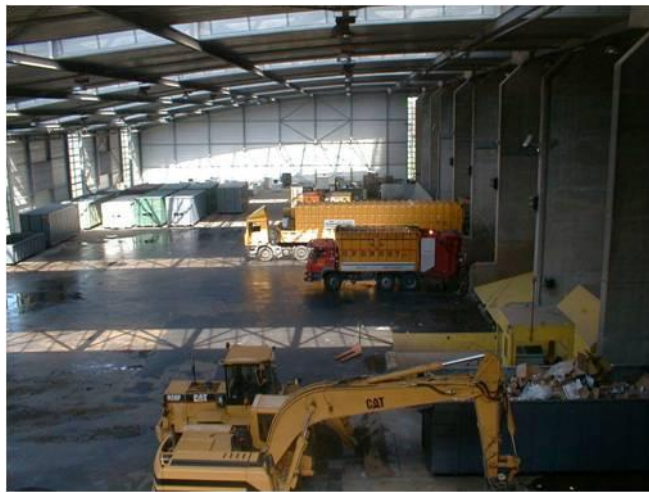
Figure 4.2: Waste reception hall of the Dutch Alkmaar incinerator
